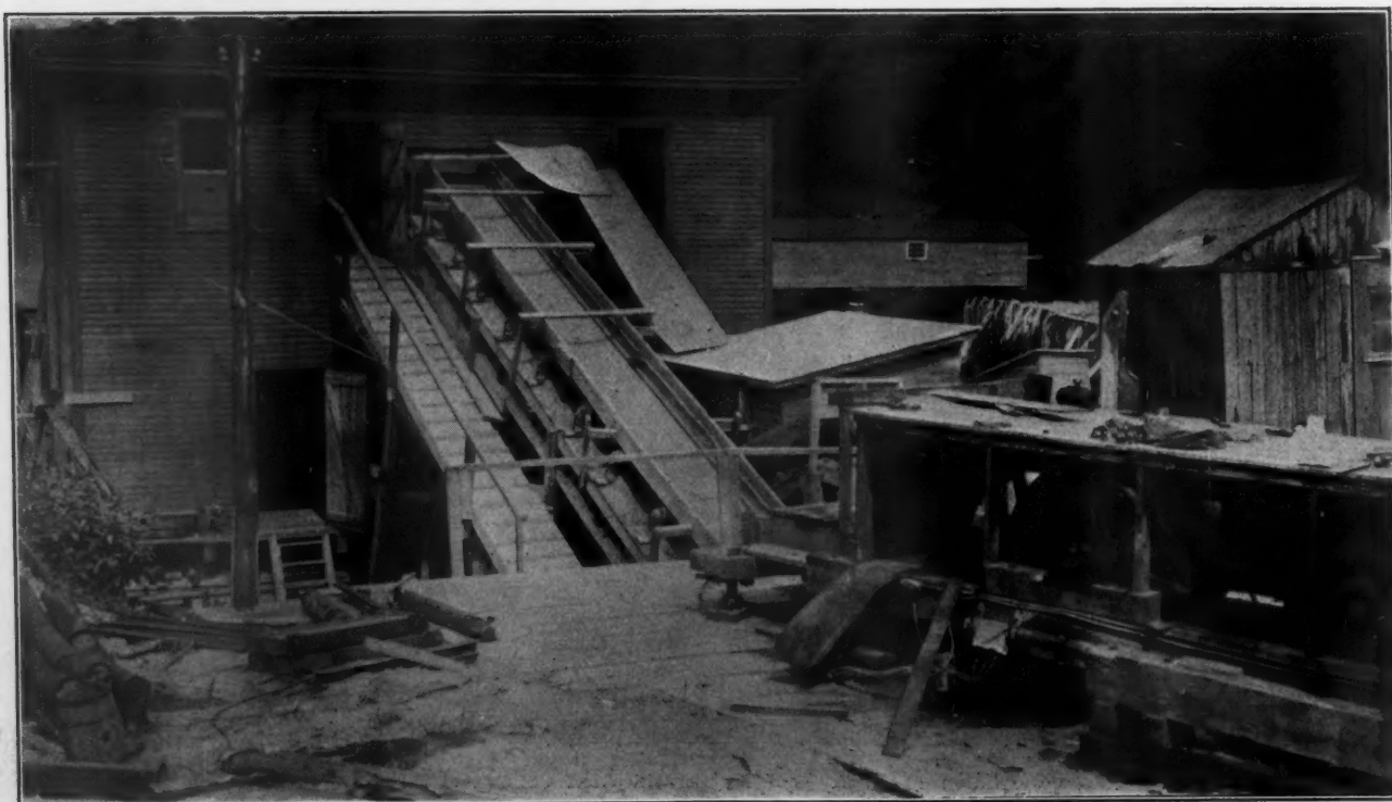
Inclined Conveyor from End of Pit Conveyor to Crushers in Building
